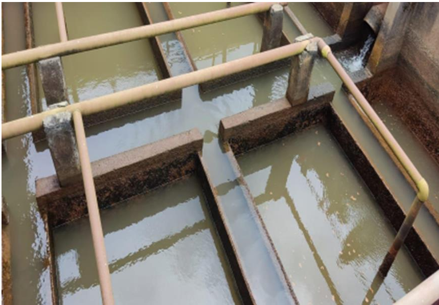
Photo No.3 Rapid Sand Filter Beds
