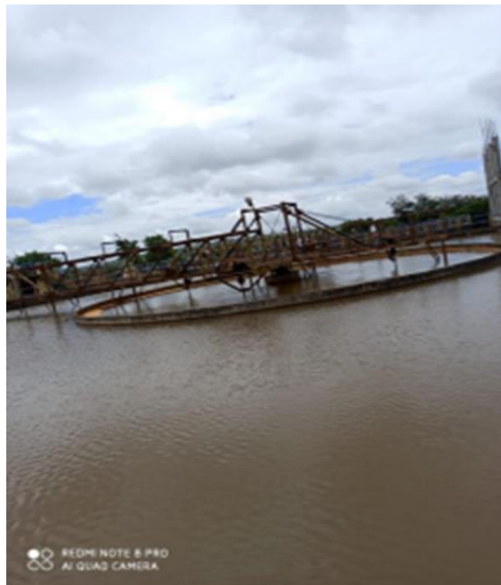
Photo No.2 Clariflocculator Tank
